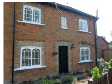
Picture 2.57 No. 12 Green Lane Cottages and its decorative brick quoin and brick surrounds to windows
