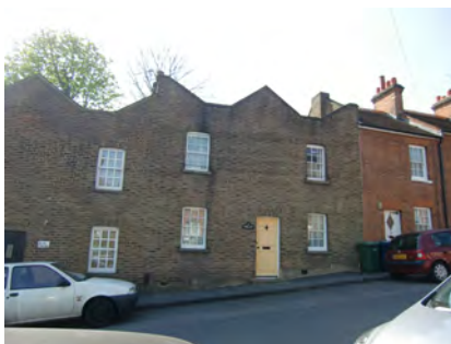
Picture 2.56 Nos. 1-4 Green Lane are unified by their angular parapet wall, also known as a Butterfly Roof
